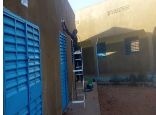
The solar system in the Lycée «Emmaus»
